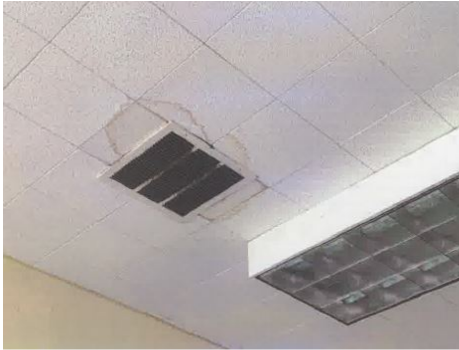
Room C - Ducting Vents
