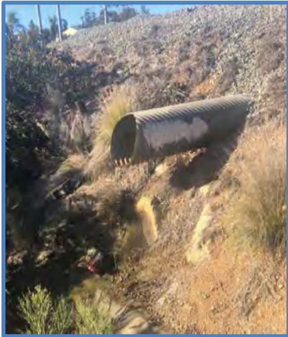
Figure 2-3: CMP conduit in the northern portion of Lemon Grove (Left). Spillway in the northern portion of Lemon Grove (Right).
